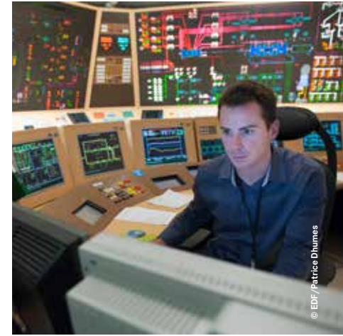
Control room in a nuclear power plant.
